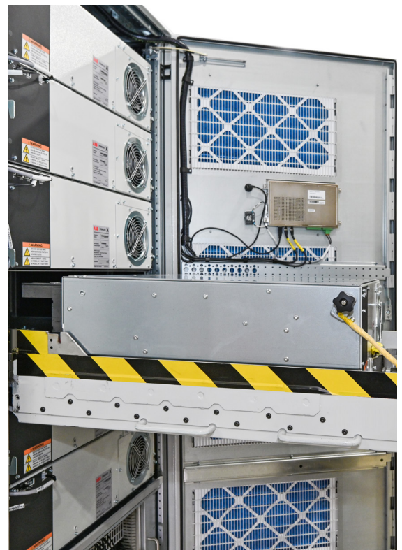
03. Power Electronics Building Block (PEBB)
